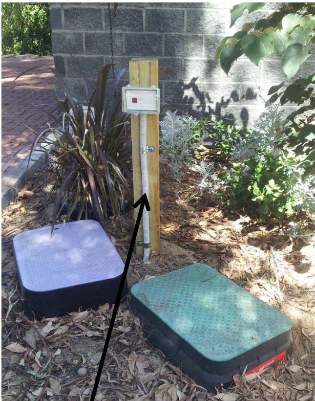
New pole with alarm plate.
